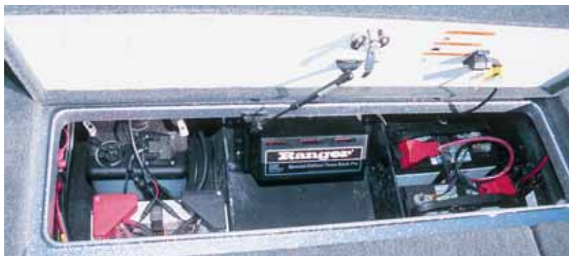
Below: The rigging is top-notch with everything in its place and the wiring neatly contained.
